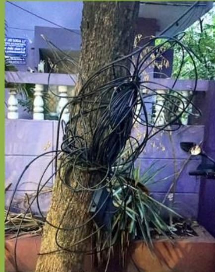
Cables tied around the branches
